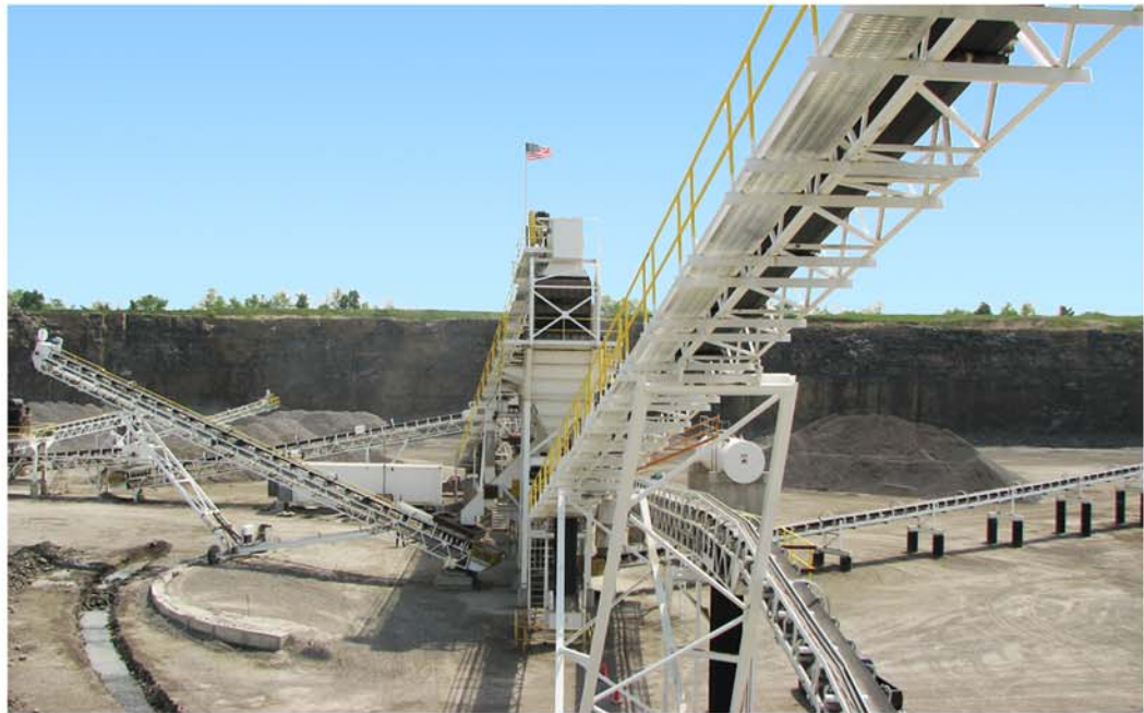
CONVEYORS IN AGGREGATE FACILITY
