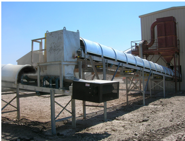
CONVEYORS HANDLING CLAY
